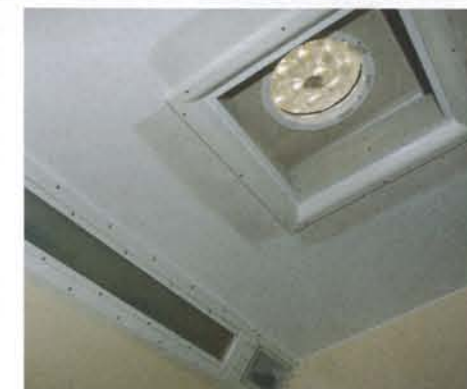
Solar tube light diffusers are fitted throughout the suite
