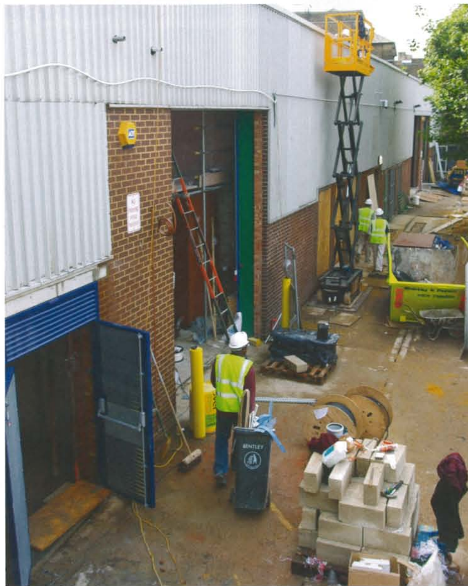
Front of the custody suite. The vehicle dock is the 2nd door from the left
